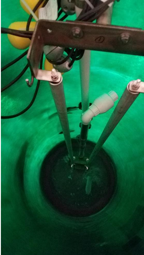
Interior of Pump Basin
